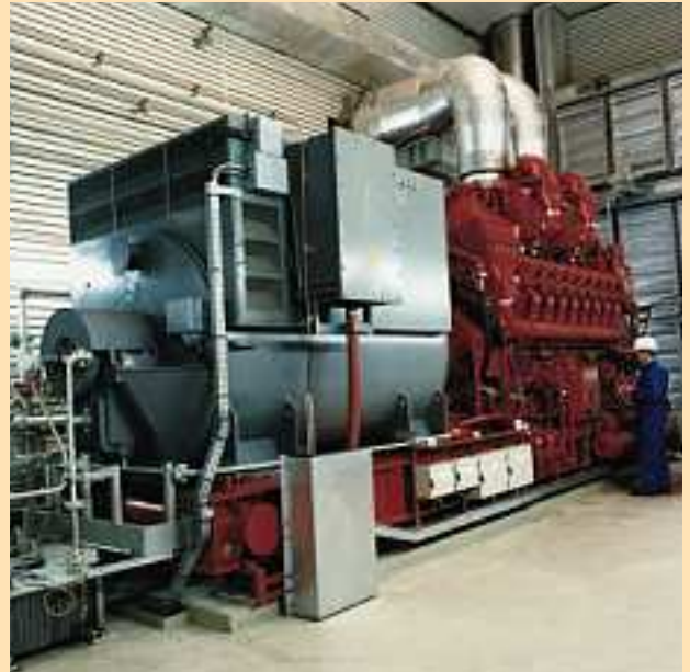
Isar-2, Germany (KONVOI, 1,300 MWe) emergency Diesel generator.
