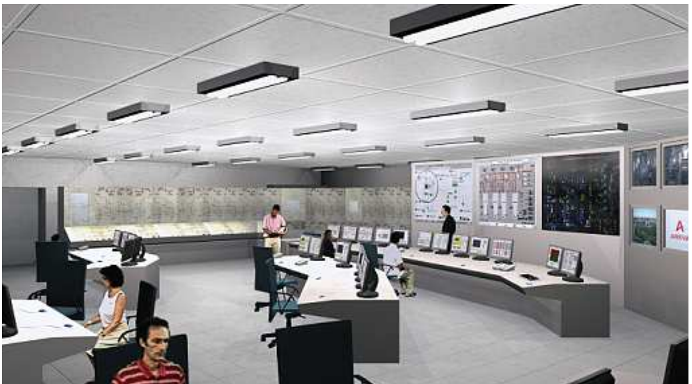
The EPR™ power plant's computerized control room features control screens providing relevant summary information on the process (computer-generated picture).
