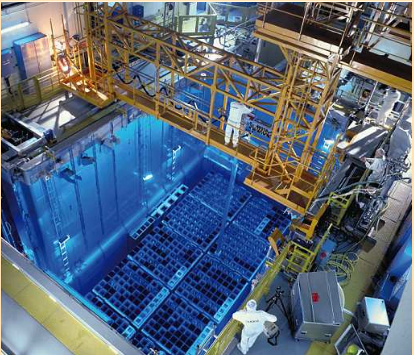
Chooz B1, France (N4, 1,500 MWe) Fuel Building.
