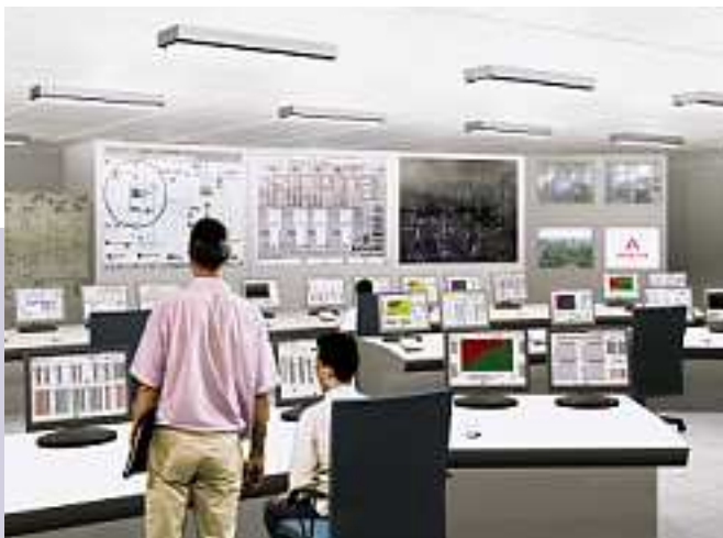
The ergonomics of the EPR™ Control Room benefits from the latest developments in human-machine interface design (computer-generated picture).
