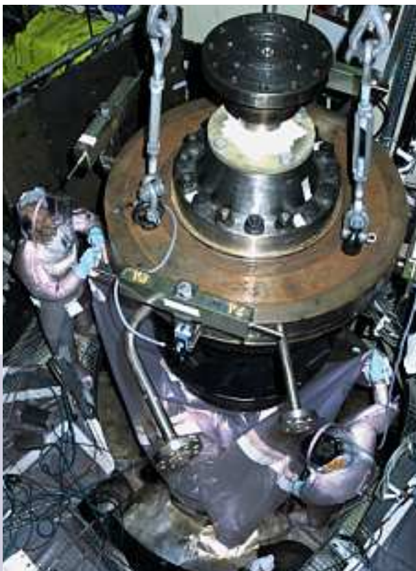
Chooz B1, France (N4, 1,500 MWe): removal of the hydraulic section of a reactor coolant pump for maintenance.
